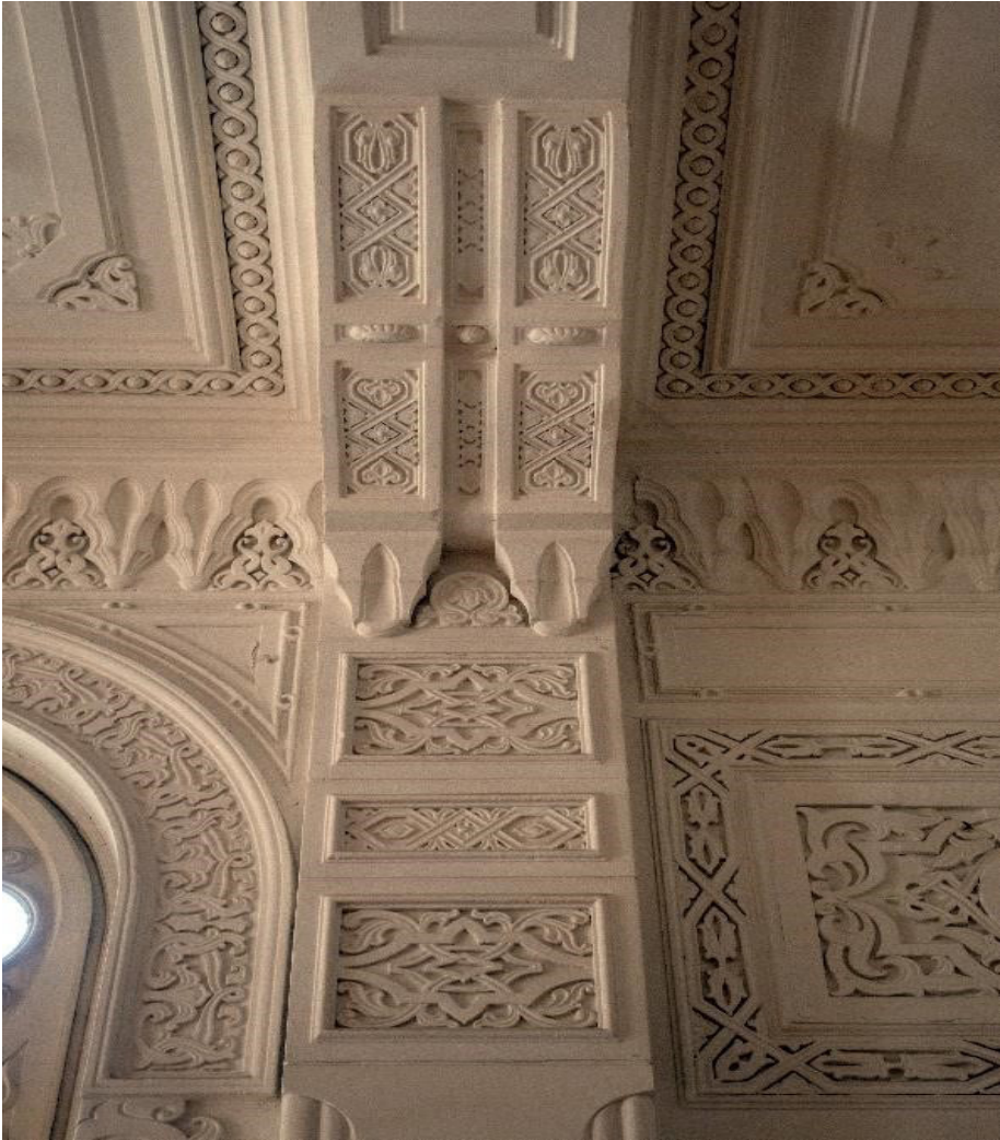
Figure 6. A detail of the plaster decoration from the ceremonial hall of the School. (Photo by Putnik and Dautović)
