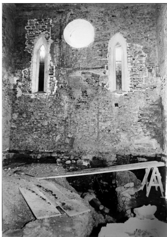
Figure 10. Eastern wall of the synagogue during excavations. Interior. Photo: The Maribor Regional Office of the IPCHS, Fond Maribor—Sinagoga.
