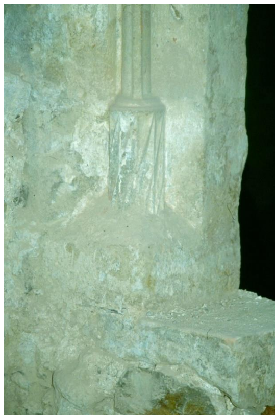
Figure 11. The entrance portal to the main hall from the west, a fragment of a rod-shape profile. Photo: The Maribor Regional Office of the IPCHS, Fond Maribor—Sinagoga.
