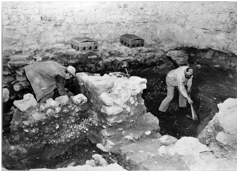
Figure 7. Unearthing of the wall foundations lying north–south, forming the western wall of a smaller building, probably the oldest synagogue phase. Interior. Photo: The Maribor Regional Office of the IPCHS, Fond Maribor—Sinagoga.
