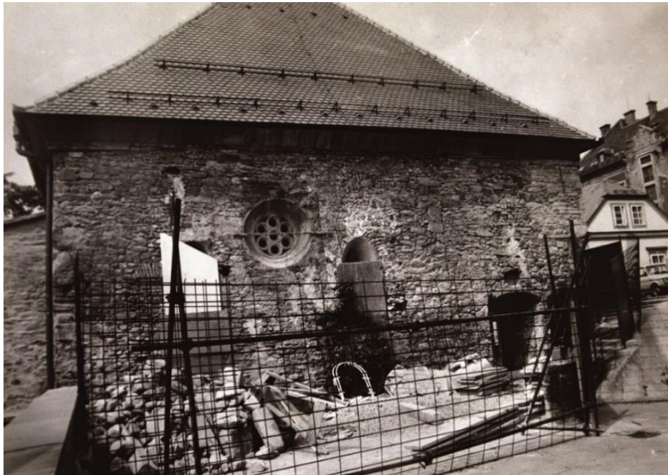
Figure 5. Eastern façade after removal of the annexed building. The openings in the wall with the rosette window and portal, leading to the lower floor of the northern annex, are clearly visible. Photo: The Maribor Regional Office of the Institute for Protection of the Cultural Heritage in Slovenia (IPCHS), Fond Maribor—Sinagoga.
