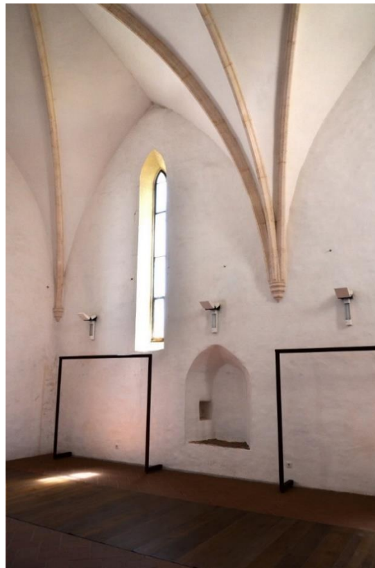
Figure 6. View of the southern wall with the niche and part of the floor covered by wooden beams. Interior. Photo: Janez Premk.
