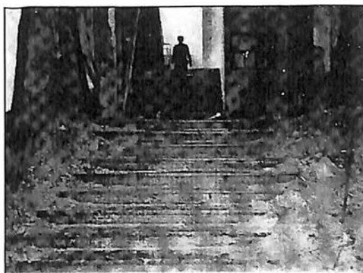
Slika 114. Oštećen ulaz i stubište zgrade židovske općine nakon eksplozije podmetnute bombe 19. kolovoza 1991. Damaged entry staircase to the building of the Jewish community in Zagreb after explosion of planted bomb on August 19, 1991
